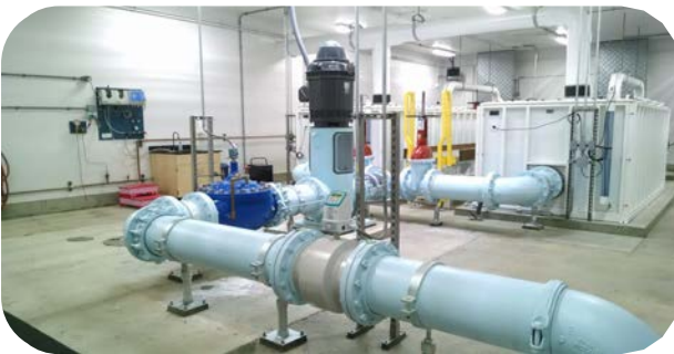
Well 5 Lowry Tanks and Booster Pump
