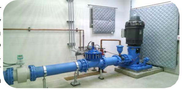
Well 5 Main Pump Room
